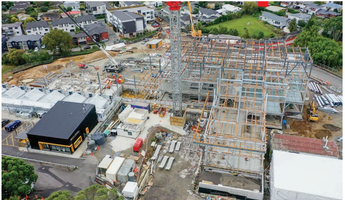
Construction of the Plant Health and Environment Capability facility for the Ministry for Primary Industries, Auckland.
